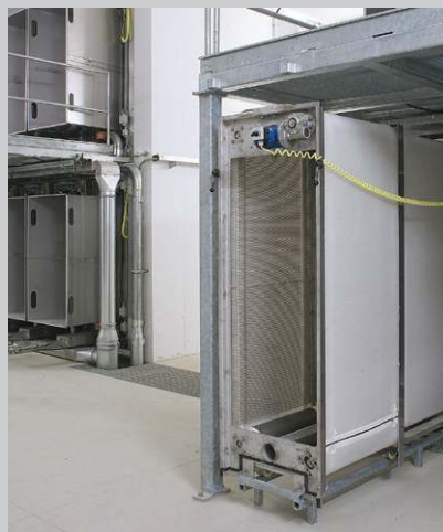
ECCO with dry cleaning system of collector
