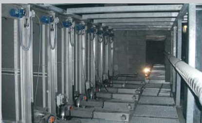
Automatic dampers for sectional cleaning
