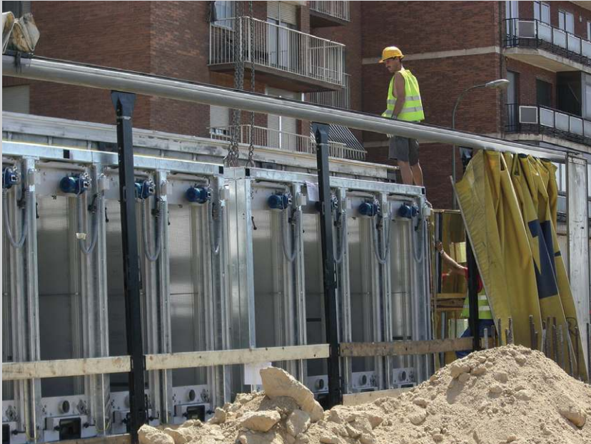
ECCO installation - Avenida Portugal
