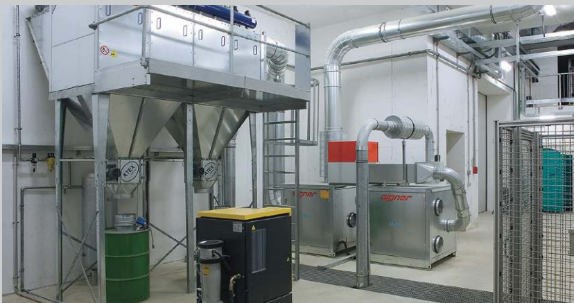
Technical room with complete equipment for cleaning, high voltage system and control system
